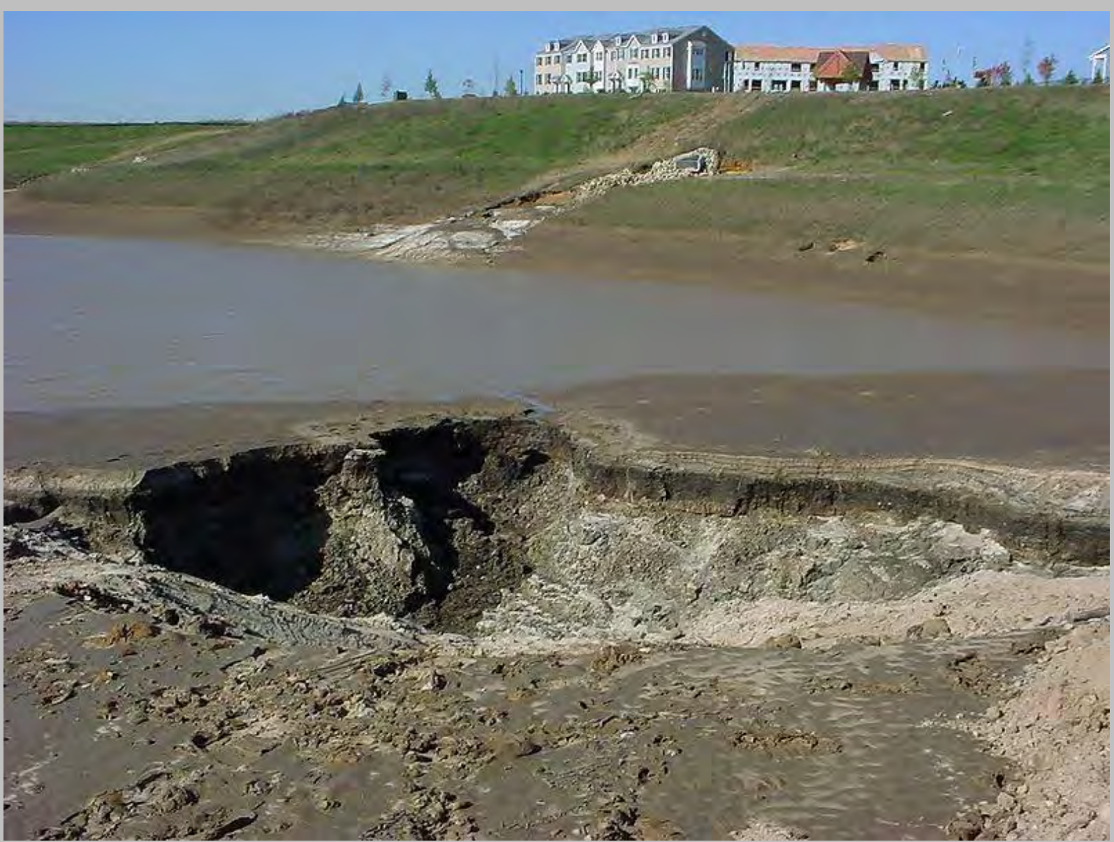
Stormwater ponds & sinkholes- sinkhole at Dancing Waters, Woodbury, MN
